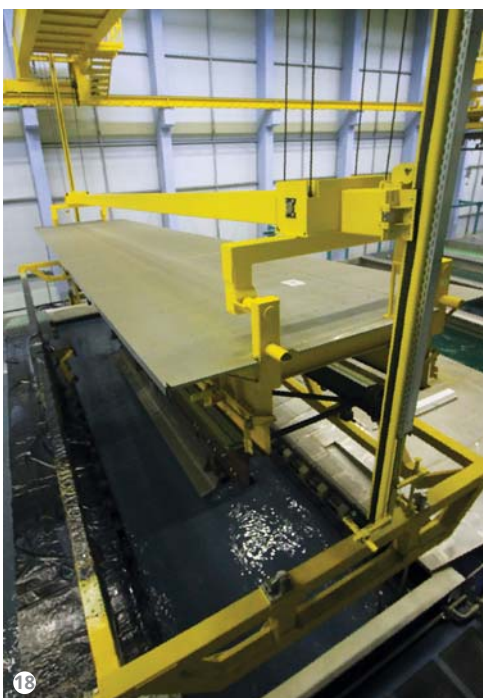
Figure 18: The cataphoresis tanks have a capacity of 250 m 3 .
