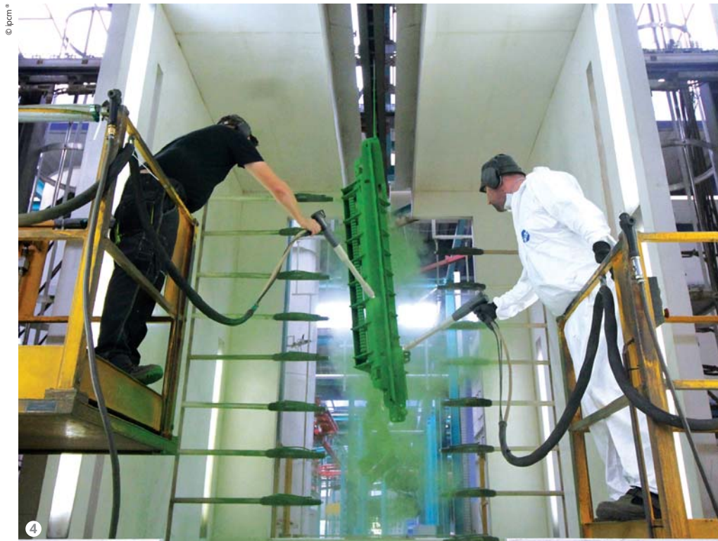
Figure 4: One of the four Wagner's powder coating booths installed on Agrostroy's Painting Line 1.
