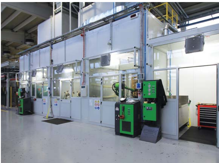
The coating booths.
