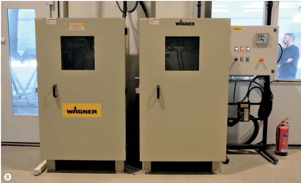
Figure 8: The paint mixing and feeding occur through the separated AquaCoat system.
