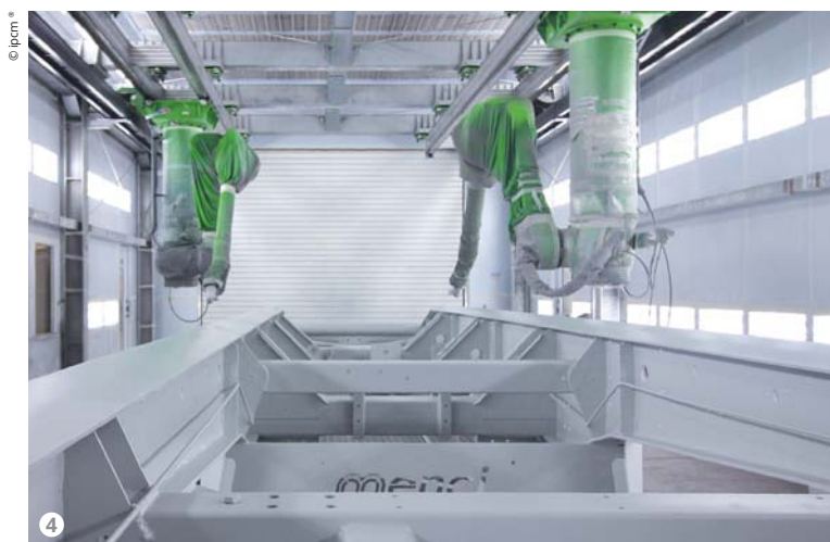
Figure 4: The two coating robots installed in the 20-metre long dry application booth.
