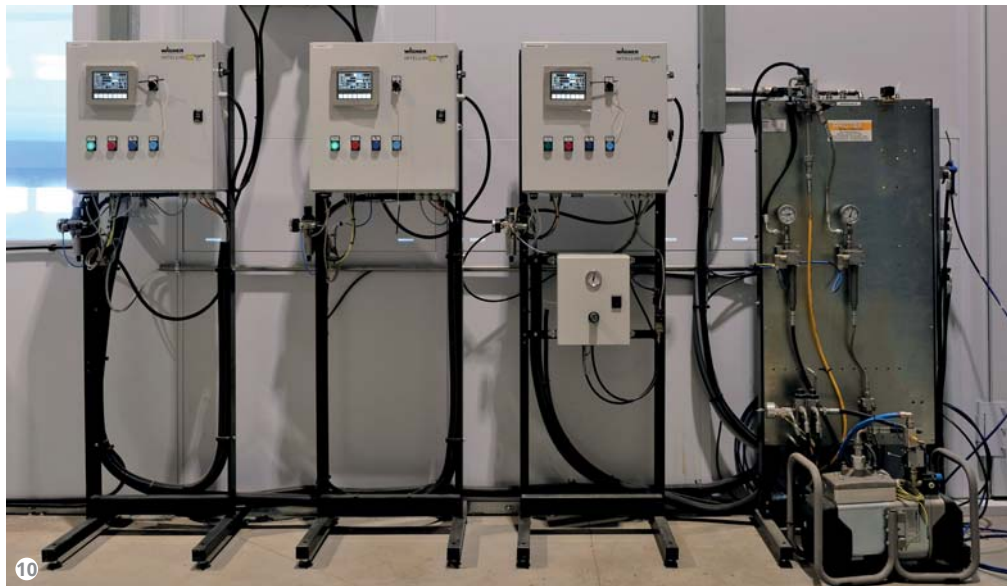
Figure 10: The control modules of the Wagner Intellimix mixers.
