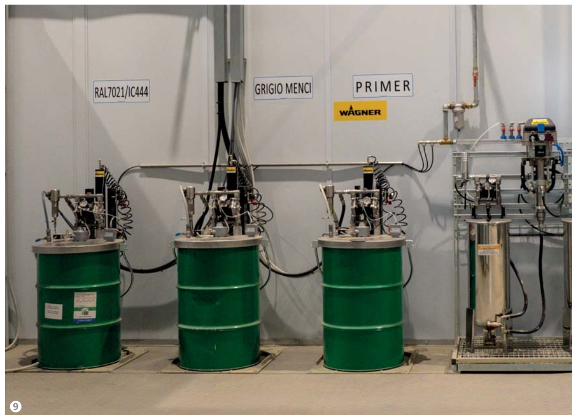
Figure 9: The coating management unit.
